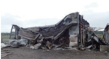
A storage battery facility after a fire
